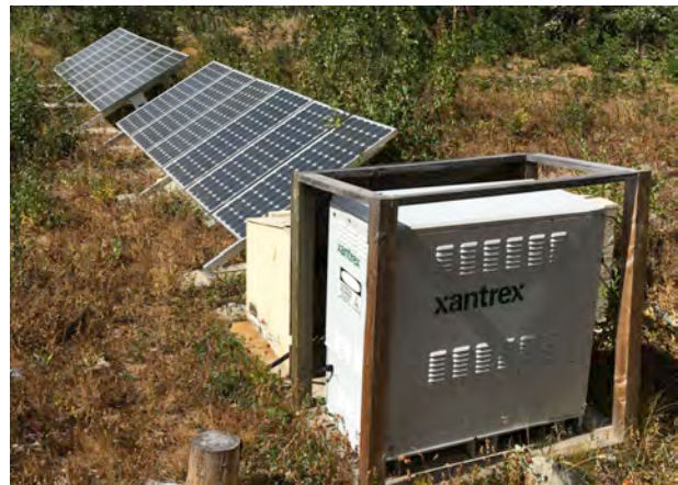
Figure 1. The original 2006 hybrid system in 2017.
